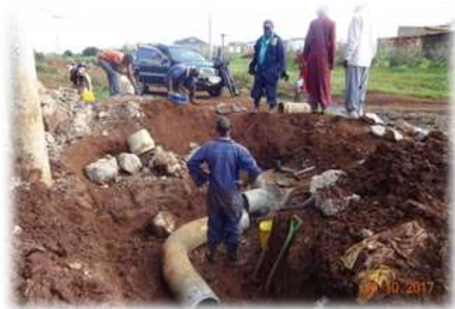
Figure 11 Water facilities in Isiolo Town
